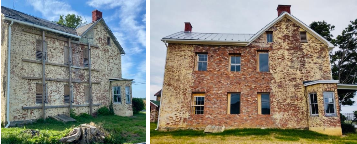
West wall of the Shafer house in June 2021 and after repairs in June 2022.
